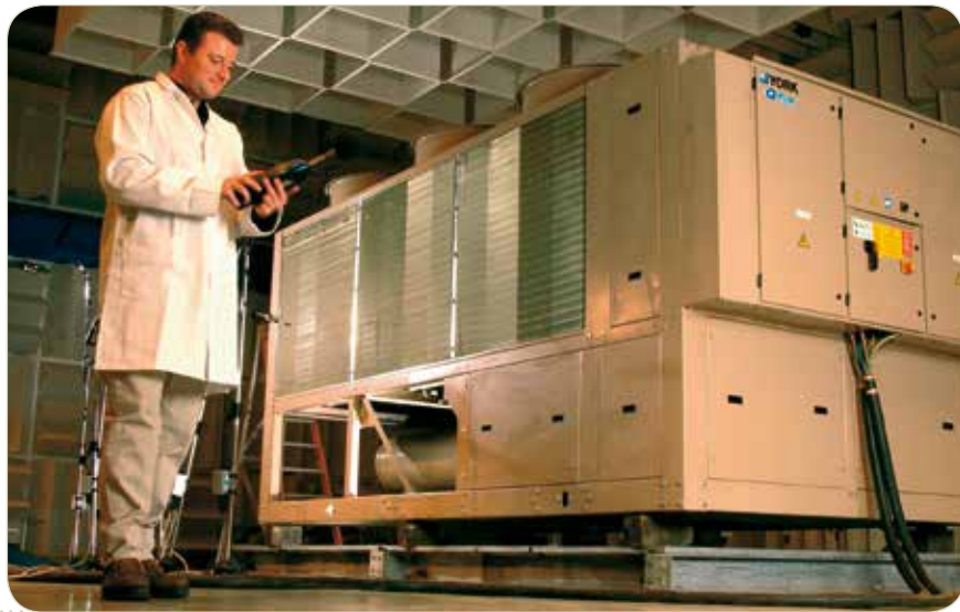
Chiller technology is continually improving with recent advances resulting in improved efficiencies over the entire load range.
